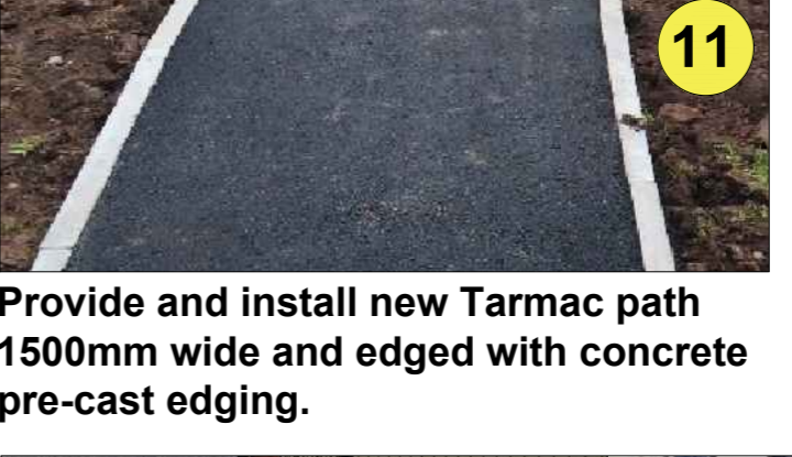
11 Provide and install new Tarmac path 1500mm wide and edged with concrete pre-cast edging.
